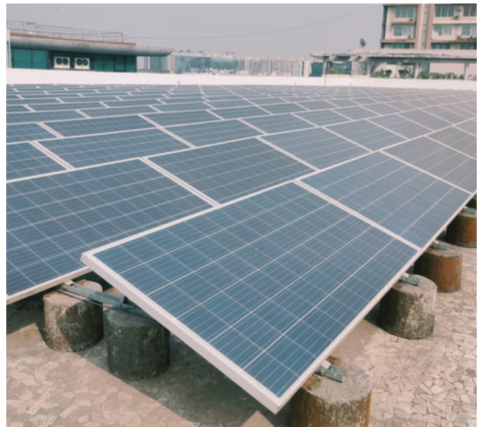
SOLAR PANELS AT PLANTS
