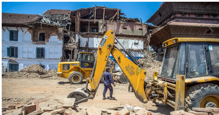
In the immediate aftermath of the earthquake, clearing operations underway in Kathmandu, Nepal, 2015. Photo: Tapash Paul/Drik.
