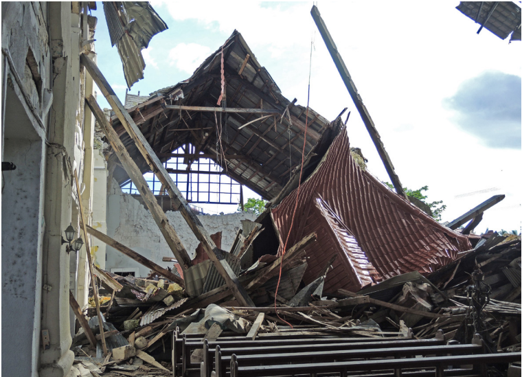
A church damaged by earthquake in Bohol, Philippines, 2013. Photo: Aparna Tandon, ICCROM.
