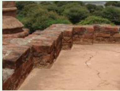
Cracks in the roof of a temple, Bagan, Myanmar, 2016. Photo: Eugénie Crété.
