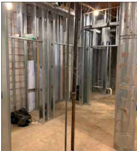
Work is being completed on the new Sacristy. Photo Courtesy: Forrester Construction
